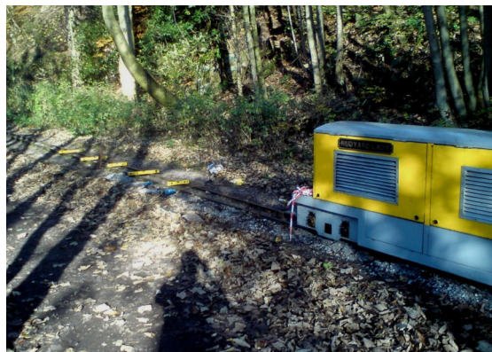
Permanent Way works taking place in the cutting; the levels are being checked prior to kango packing ballast under the sleepers, 17-11-2011. Ed
